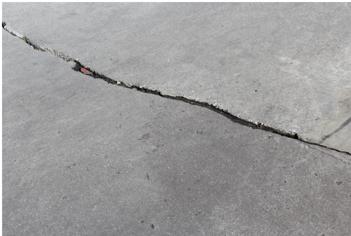
Picture of Skate Park Crack
